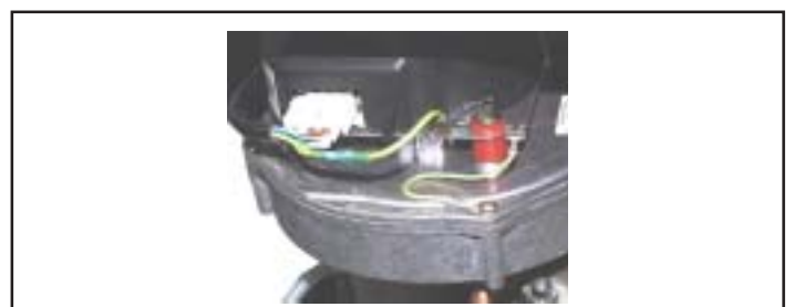
Fan supply and earth cable
