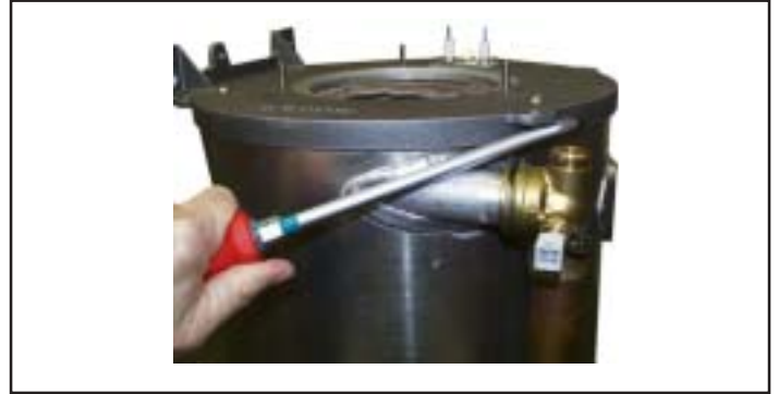
Releasing the lid from the combustion chamber
